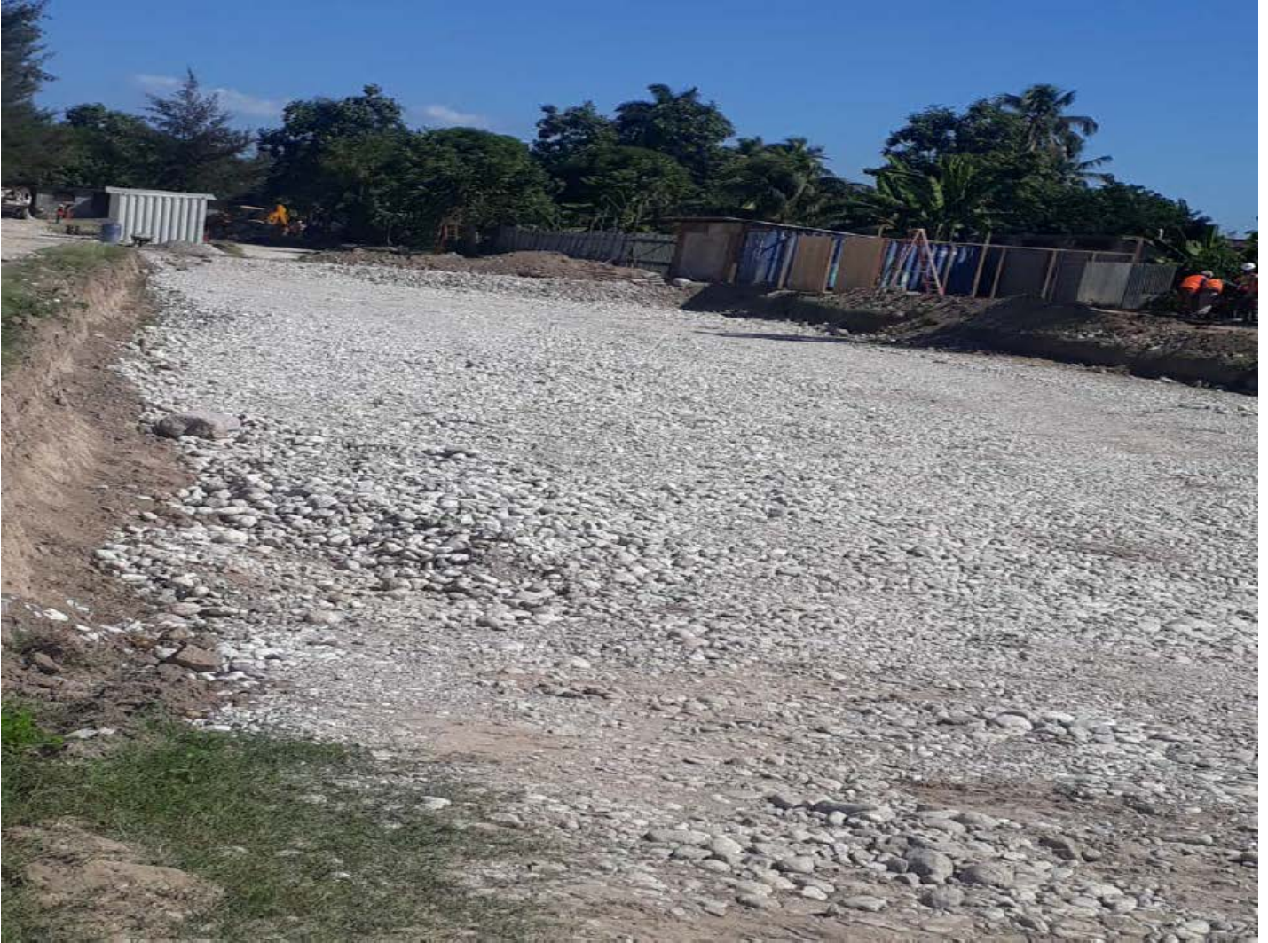
Second layer of backfill in classrooms awaiting compaction test by the building laboratory (LNBTP)
